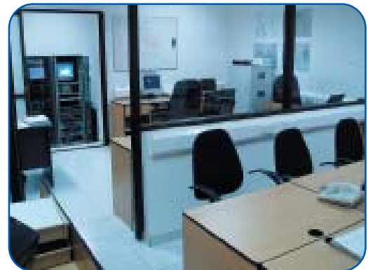
NWSC Computer Room (Headquarters)
