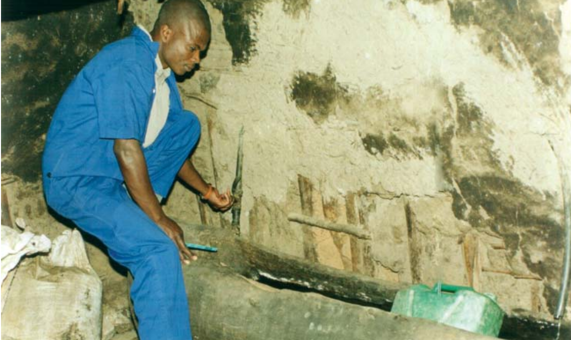
Unearthing a by pass: Illegal diversion of this nature causes water losses to the Corporation
