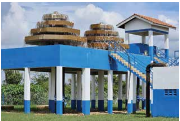
Kyankwanzi Water Treatment Plant
