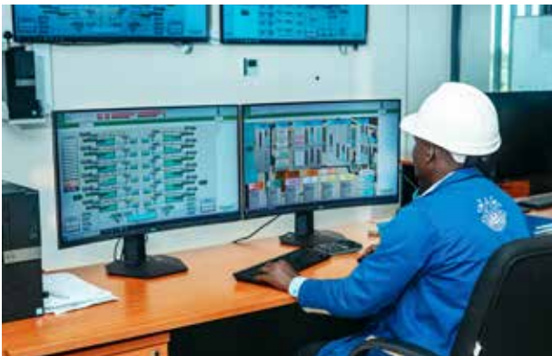
NWSC Staff smooth plant operations through computerised plant Systems (SCADA)
