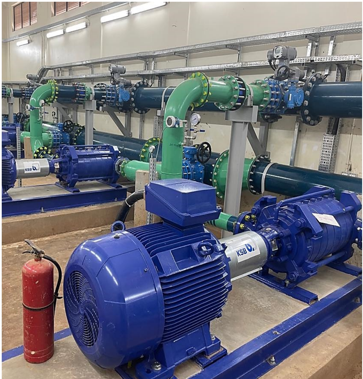
Pumps at Gulu water treatment project constructed to improve water supply services to Gulu City (10 million litres/day)
