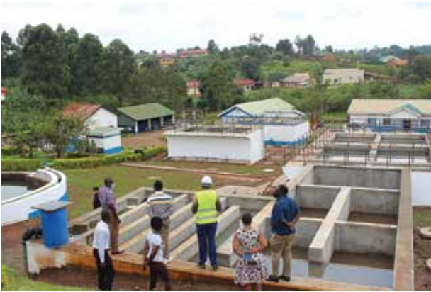
Fort Portal WTP under the Fort Portal Water Improvement Project
