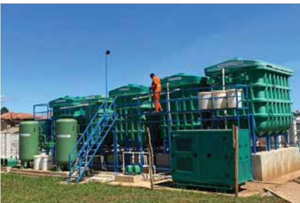
New Kirundi Compact Sewerage Treatment Plant
