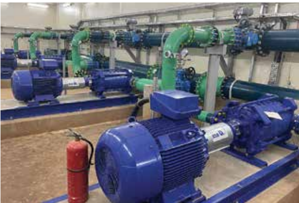
Gulu Water Treatment Plant
