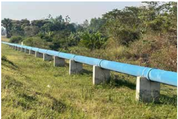
Karuma Transmission Line
